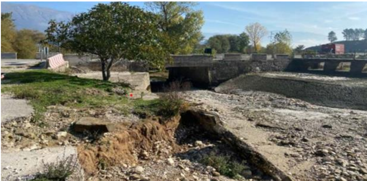
Figure 5: Damages to the structures and the lake bed after the high water levels.
